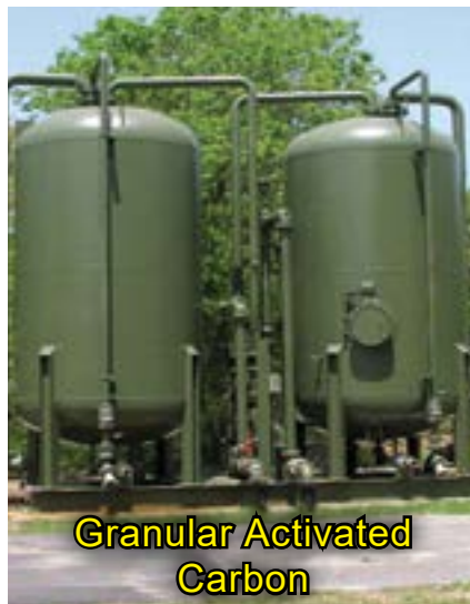
Ion Exchange Filters for Nitrate Removal
